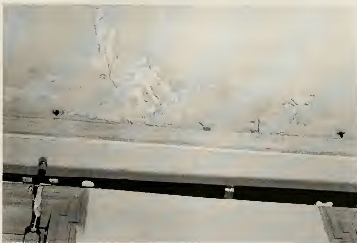
Figure 30 Deterioration of Ceiling Plaster Due to Inappropriate Mechanical System, 1998 Photograph by Author
